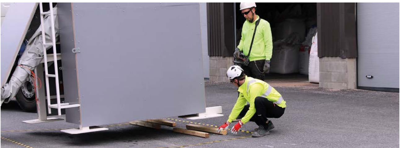
The silo is assembled at a two-degree angle in the direction of the pipe mixer.
